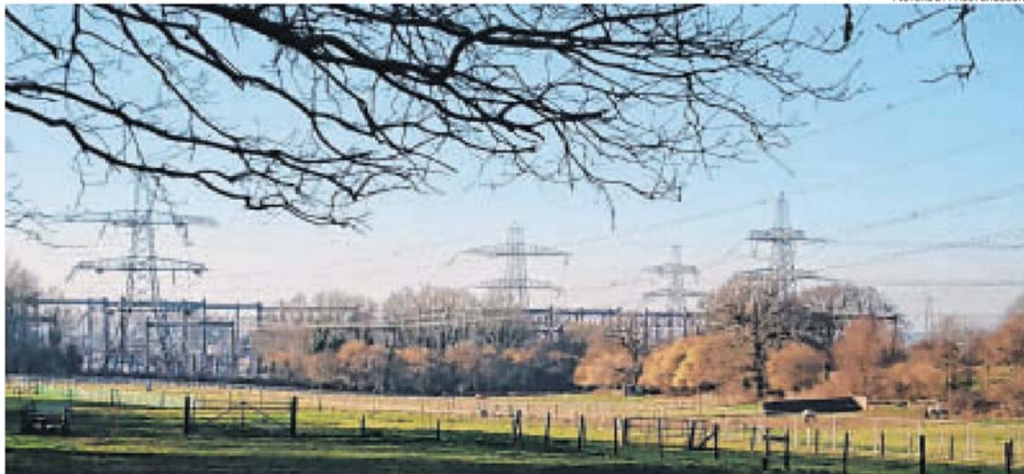
Land west of the Lovedeane substation, seen here from the north, has been earmarked by Aquind for a converter station.
